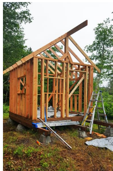
Example of Bnnkie under construction as of last Spring. It will have sleeping lofts at both ends and a futon bunkbed, electricity and small heater inside. We hope to have two by end of August.
